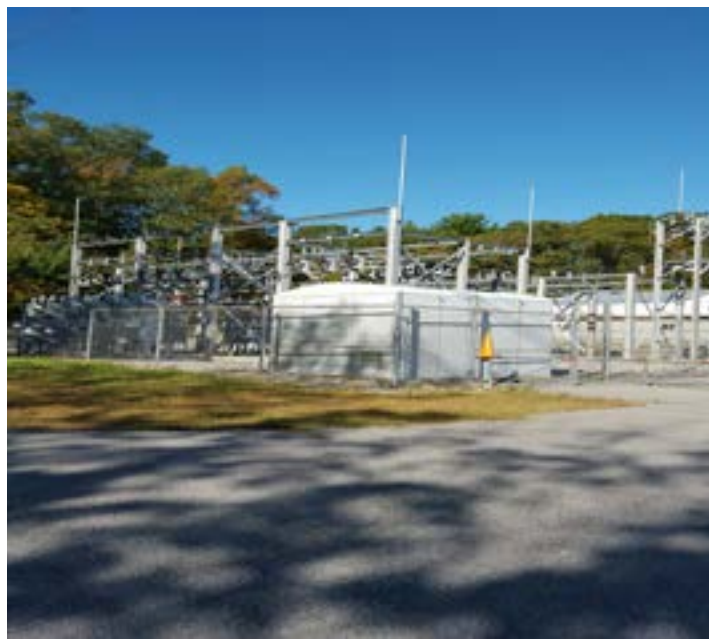
$2.1 million high-voltage substation built by AFSCME members.
